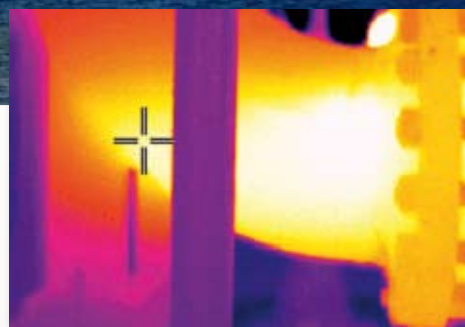
Infrared image of an oil installation.
